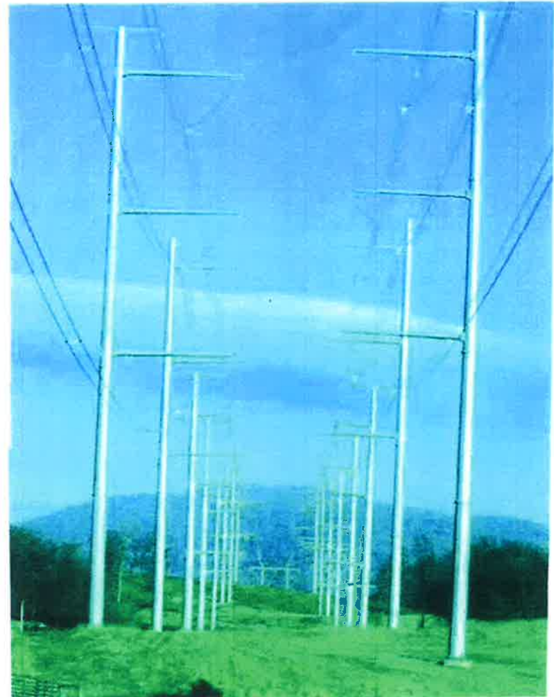
Changes in towers, wires, etc. adding 2 nd 500kV line in easement pursuant to broad language (below) in form right of way agreement signed by owner to settle condemnation proceeding
